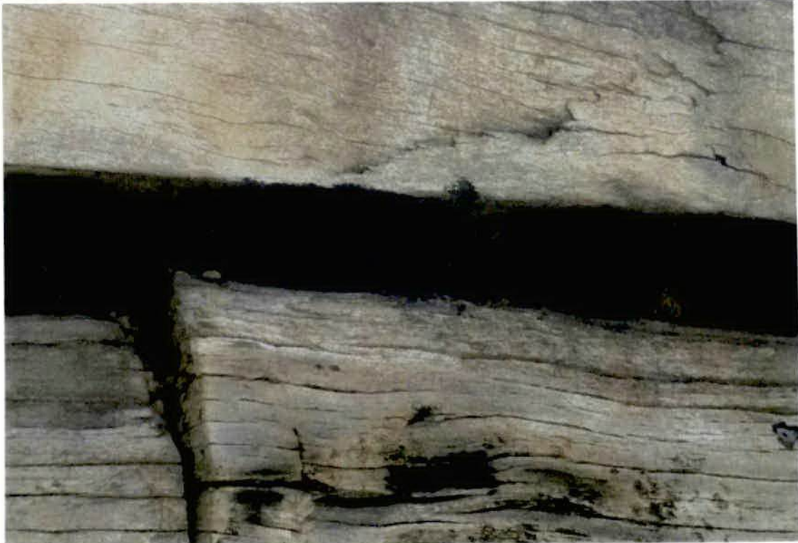
Photo No. 21: Span 3, 6 unsound deck ends from pier 3 towards abutment 2. (Taken: 24-Jan-2018)
