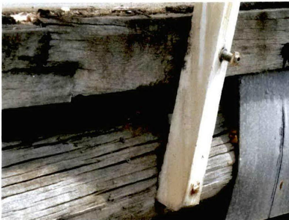
Audit Photo No. 2: Span 1 RHS, deck ends intermittently U/S. (Taken: 15-Mar-2018)
