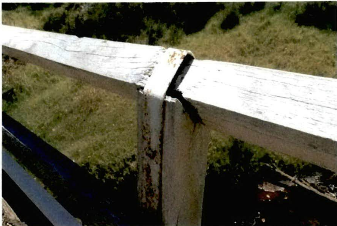
Photo No. 18: Right hand side top rail, above pier 1 damaged. (Taken: 24-Jan-2018)
