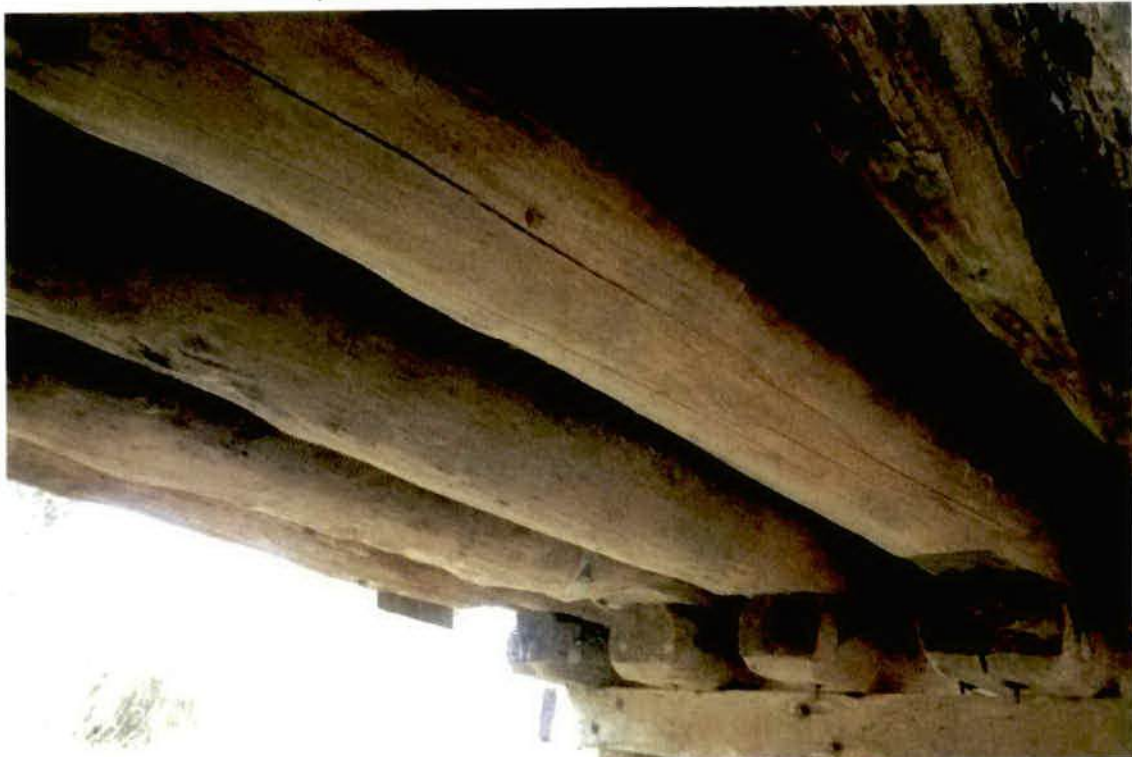
Photo No. 10: Stringer layout in span 3 from left hand side. (Taken: 24-Jan-2018)
