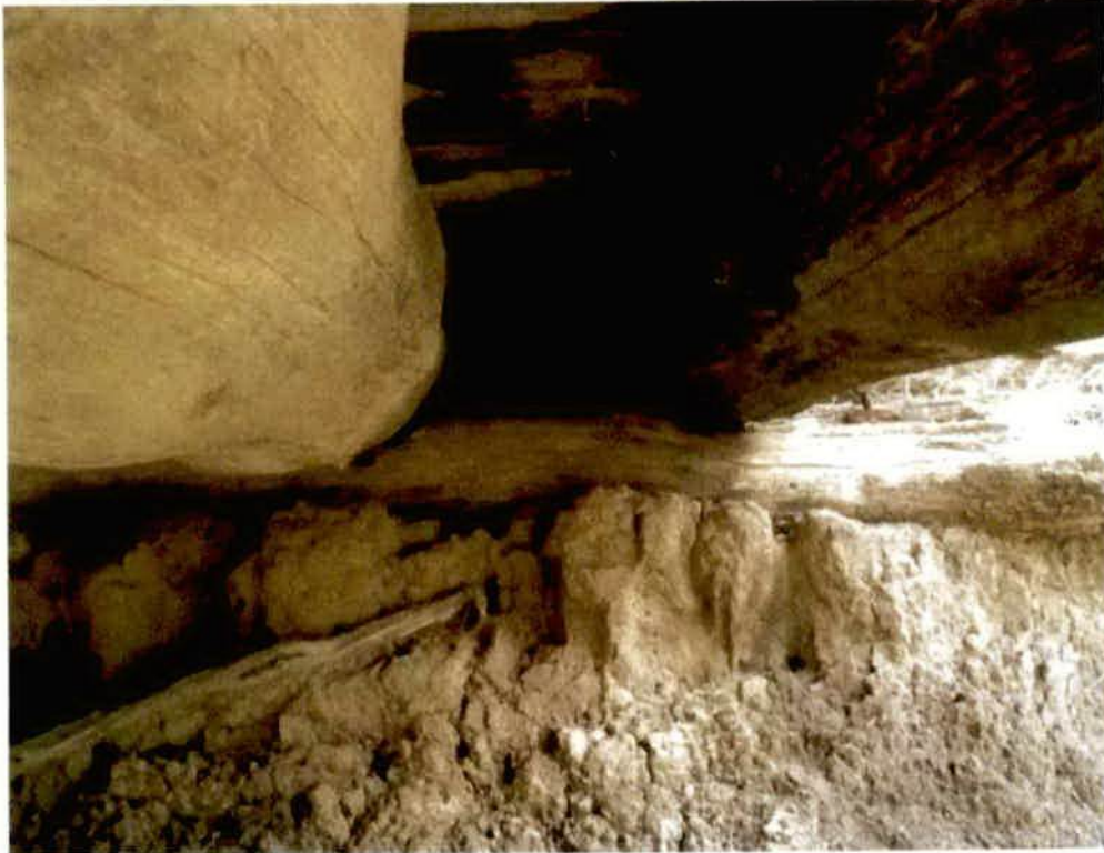
Audit Photo No. 3: Abutment 2 bedlog RHS, scour is beginning to compromise footing. (Taken: 15-Mar-2018)
