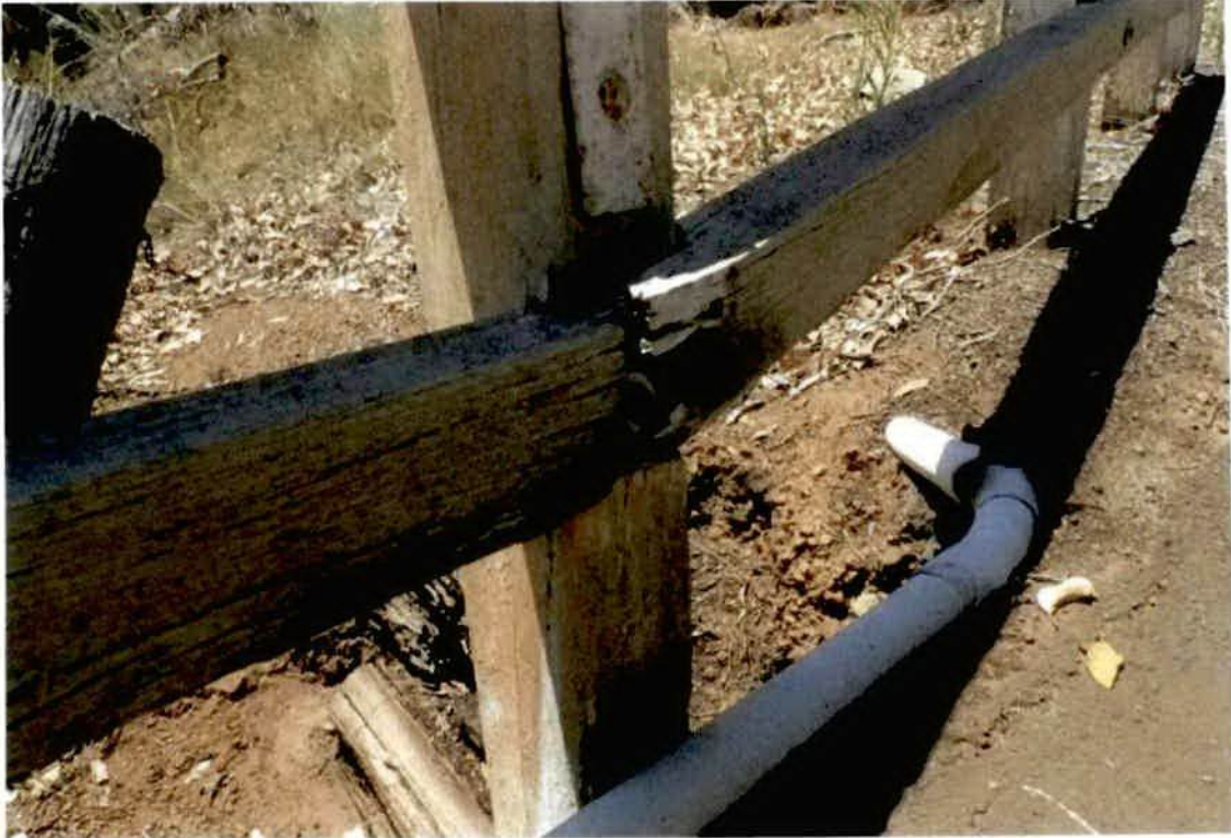
Photo No. 17: Right hand side rail damaged at corner, abutment 1. (Taken: 24-Jan-2018)
