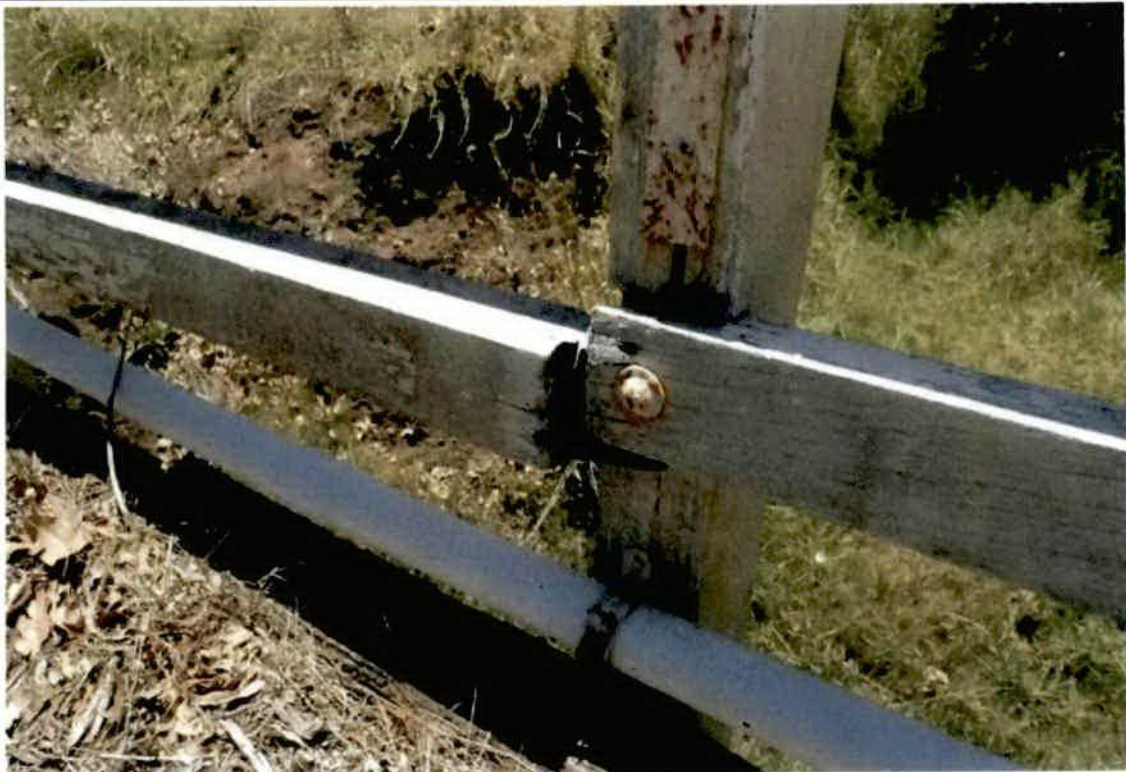
Photo No. 19: Right hand side bottom rail, abutment 2 end damaged. (Taken: 24-Jan-2018)
