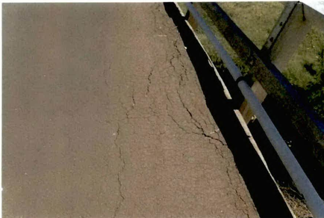
Photo No. 14: Bitumen seal cracking along kerb line from abutment 1. (Taken: 24-Jan-2018)
