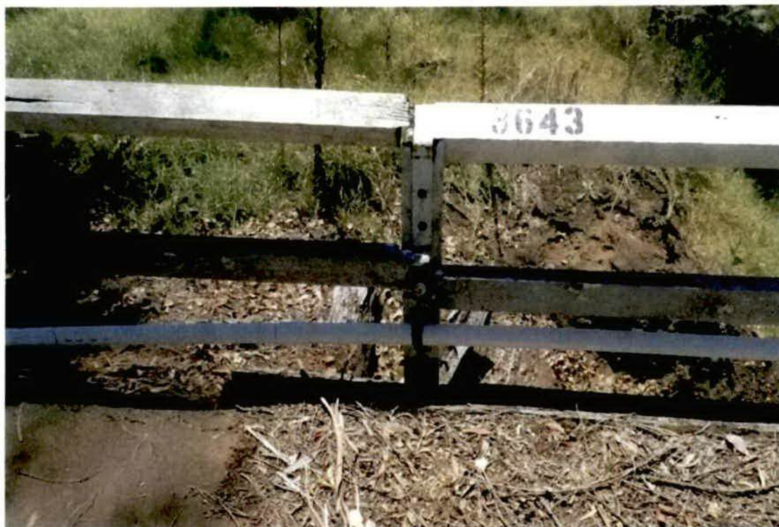
Photo No. 16: Abutment 2 right hand side barrier, broken. (Taken: 24-Jan-2018)
